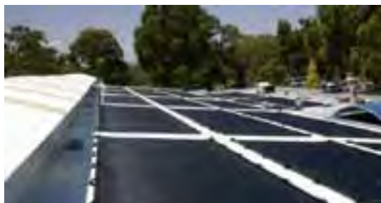
Image 14-A: Belmont Oasis Leisure Centre solar water heater
