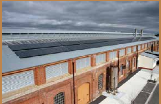
Image 13-B: Midland Foundry's 60kW solar PV system
